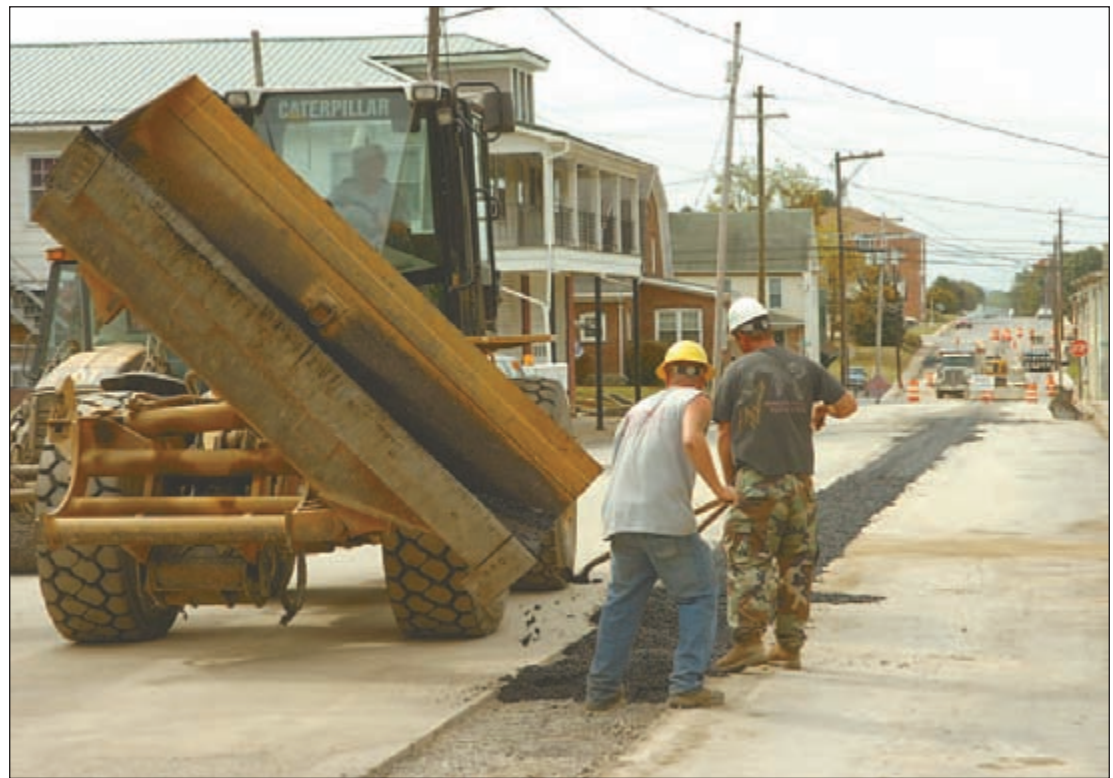
Charles E. Brake Co. employees work Tuesday on North First Street near the intersection of Lincoln Way West installing McConnellsburg's new 12-inch water main. The project is expected to be completed in November. Some streets in town will be closed as work progresses.
