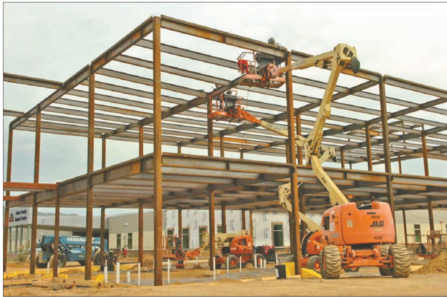
The framework of Fulton County Medical Center's 16,000-square-foot patient services addition nears completion Tuesday morning. Hospital officials invite the public to a topping out ceremony on Tuesday, October 13, to sign the structure's final beam and watch as it is set in place. The Medical Center says its new addition will be ready for patients in June 2010.
