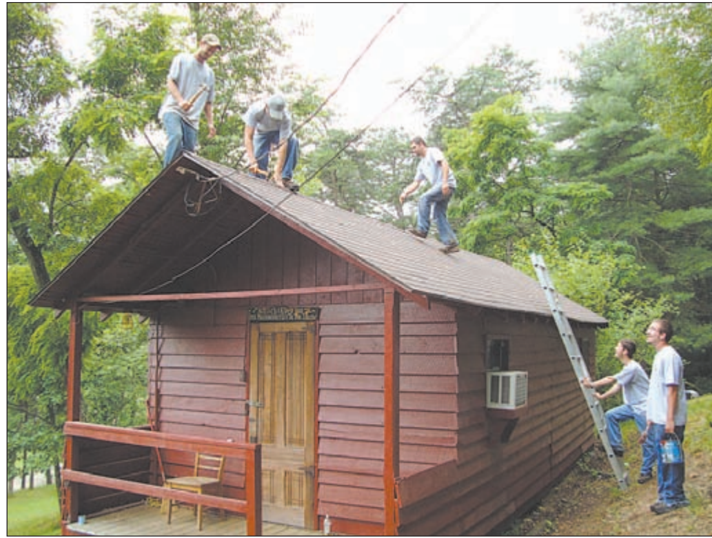
Sinoquipe Scout Reservation has seen many improvements and general maintenance projects completed over the summer as a result of a work crew funded by the American Recovery and Reinvestment Act and Southern Alleghenies Workforce Investment Board. Above, the crew puts the finishing touches on cabin shingles.
