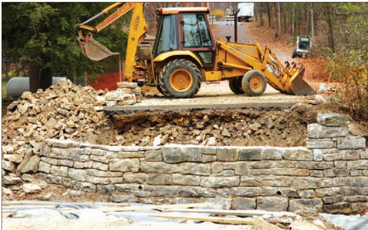
Bridge abutments on this bridge at Cowans Gap State Park were built by the Civilian Conservation Corps workers in the early 1930s. Although the bridge deck is being replaced, the abutments will remain and will be repointed. The bridge, located at the southern end of the lake, leads to Campground "B."
